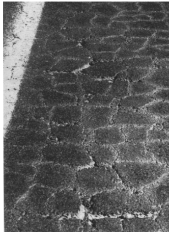
Fatigue cracking [Source: Jackson, 1988]
