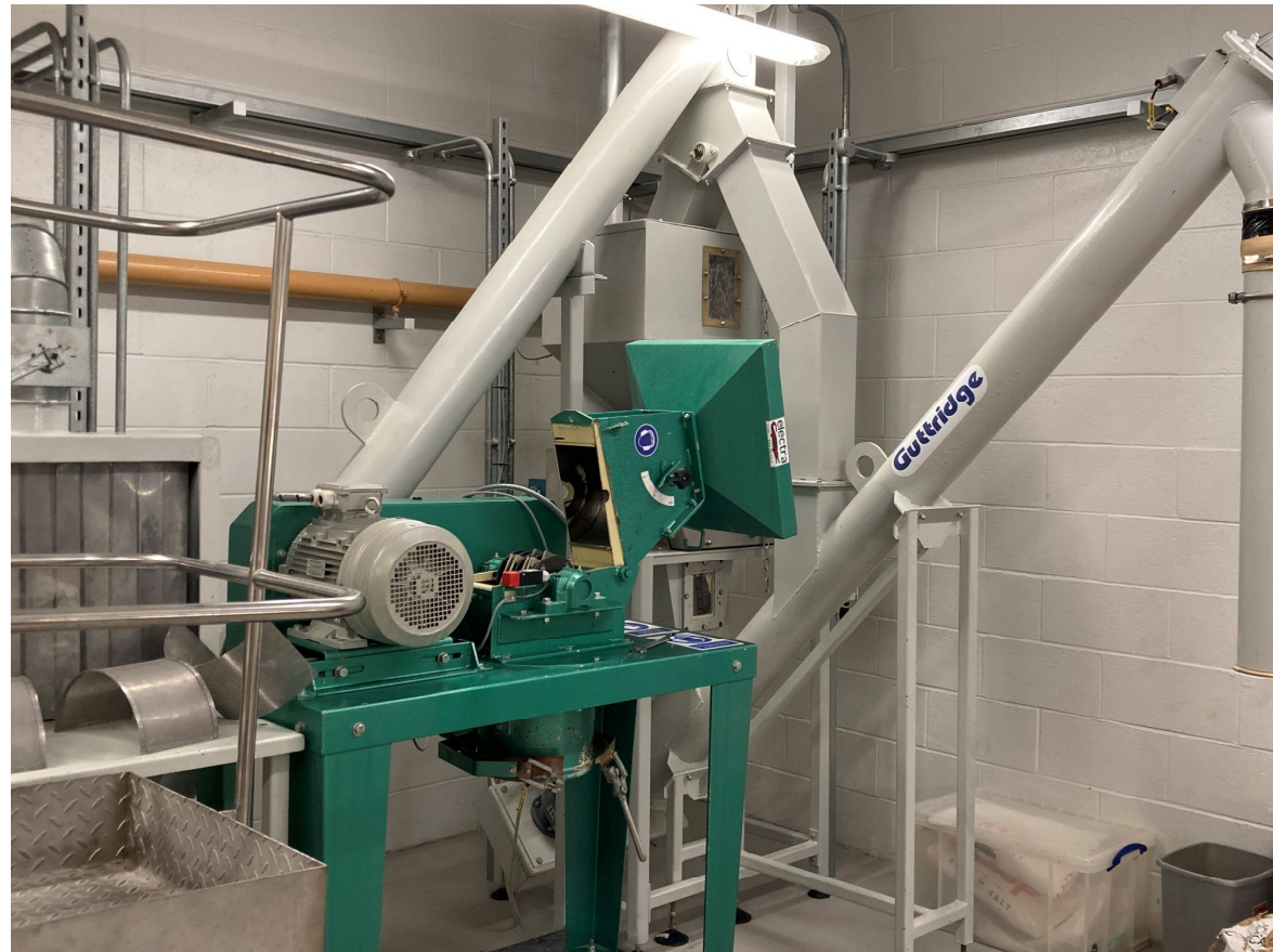
Hammer mill (green/foreground) & 2-roll mill (grey/ background)
