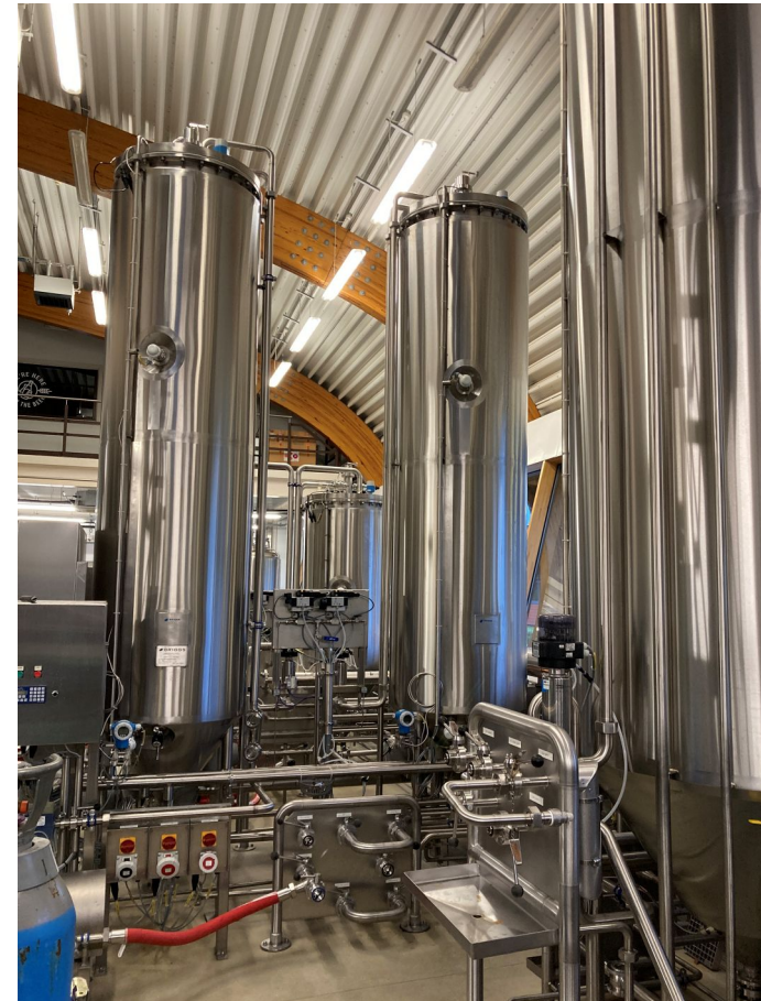
FV tank farm
