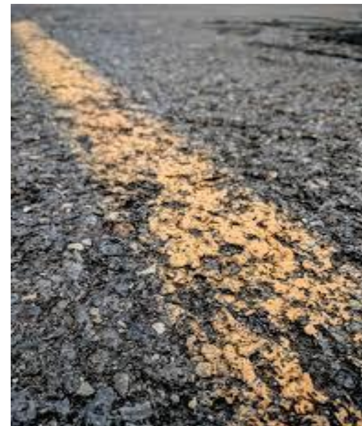
Figure 1. Raveling on an asphalt surface [3]
