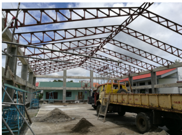
(R). Construction of a gymnasium in Tacloban. (Photo taken by Joy Spiliopoulos, June 2017)
