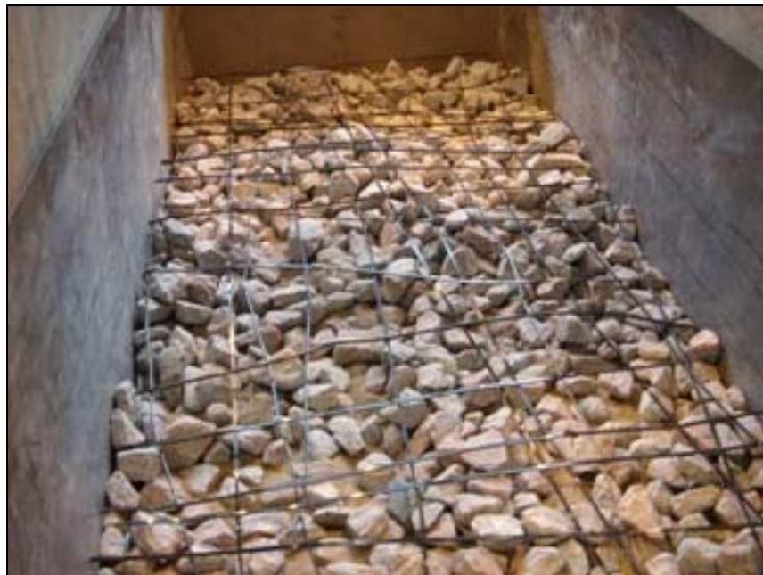
Figure 4.29 Broken grid junctions
