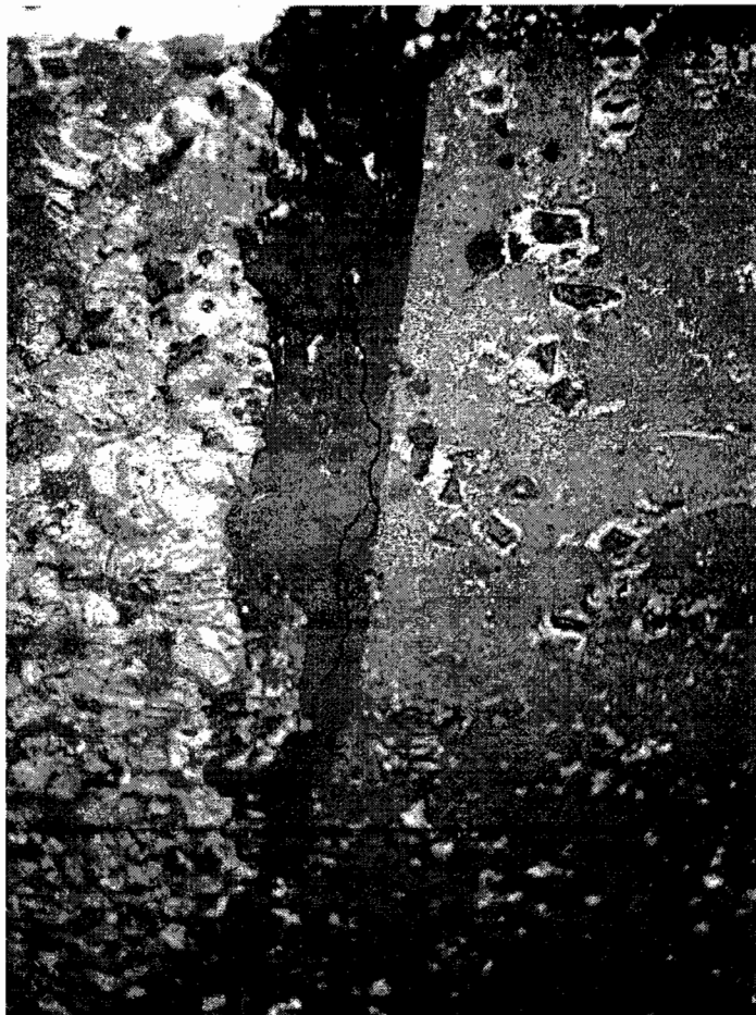
Figure 3.7: Cracks along the bitumen sealing on the leading edge. Traffic flows from left to right
