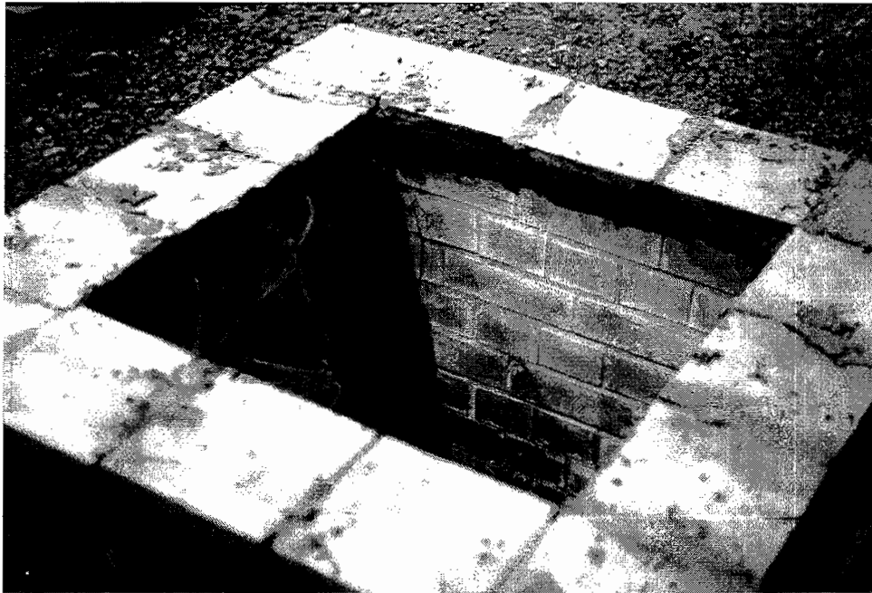
Figure C.7: Installation of quarry tile configuration. Wires connected to instruments in the bedding
