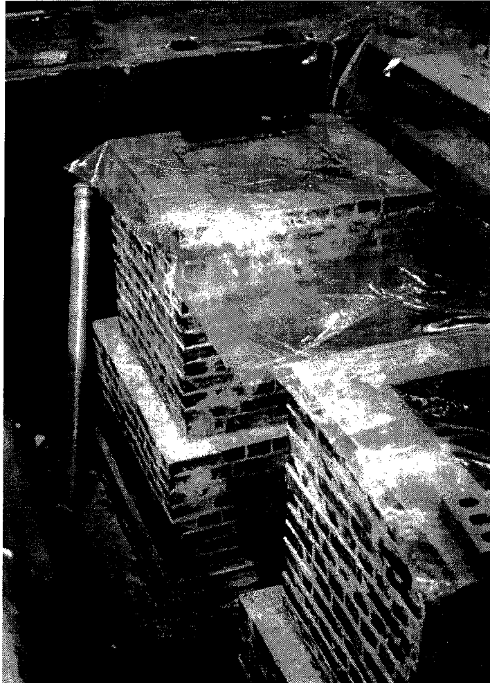
Figure C.4: Completed manhole chambers. Pipes later used as access conduit for instrument wires
