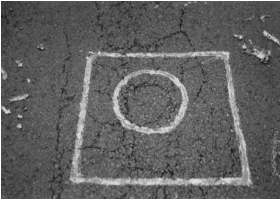
Plate 3.2 Area of 'alligator-type' cracking (Site 6)
