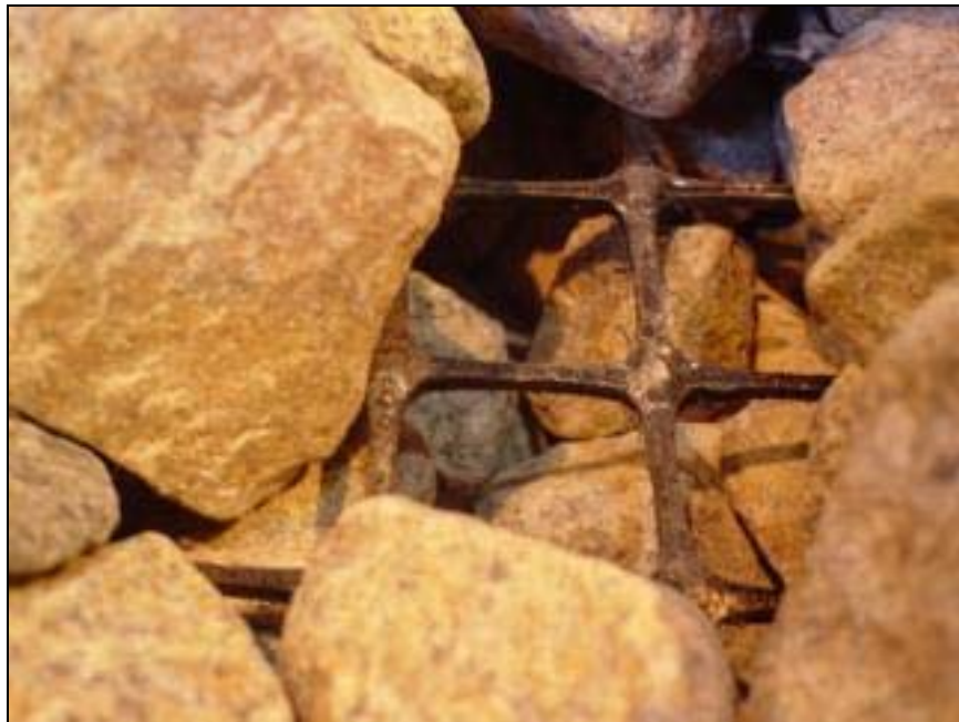
Figure 4.15 Shear failure plane in 40-32 (A/B: 0.8) reinforced CET
