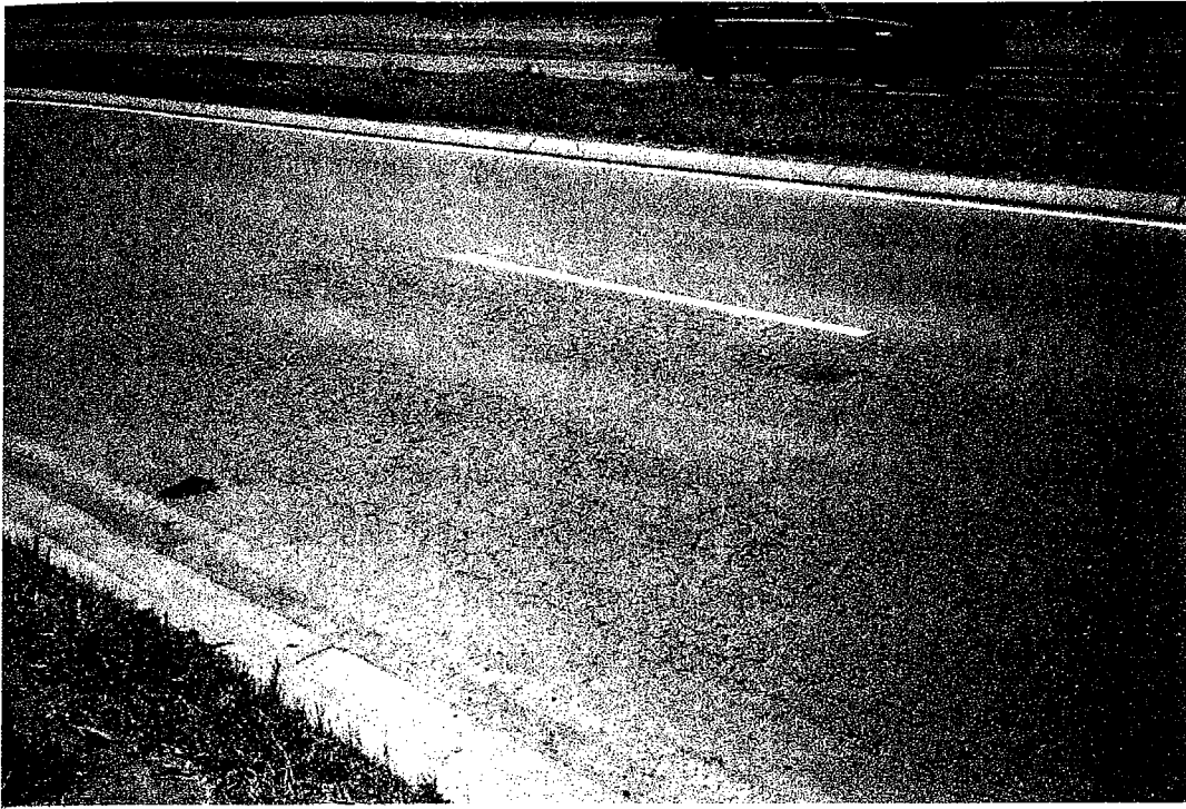
FIGURE 10.11: CRAZING OF SURFACING (CH. 1.1KM, WESTBOUND CW, OUTER LANE – TYPE 2 PAVEMENT)
